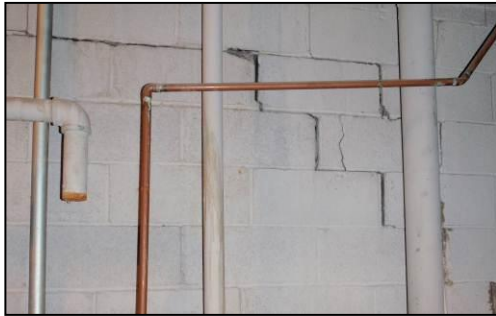
Cracked loadbearing wall that was fixed through an emergent project
