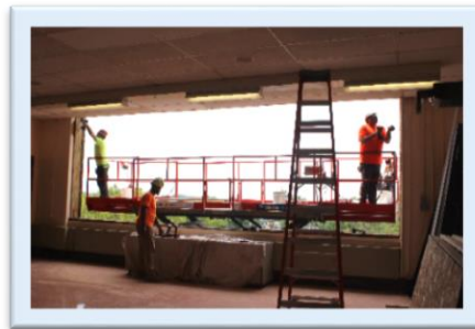
Workers reconstructing window frames to allow for the installation of new windows.
