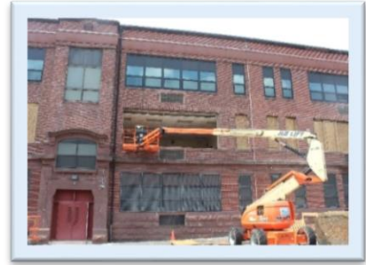
Camden Cramer Elementary School - view of original windows, replacement work, and new windows.
